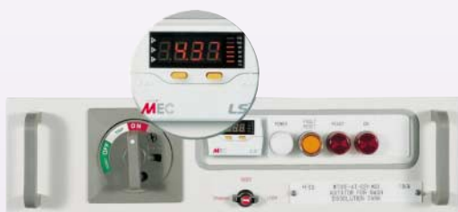
*Fig. (D-EMPR in the MCC unit)
